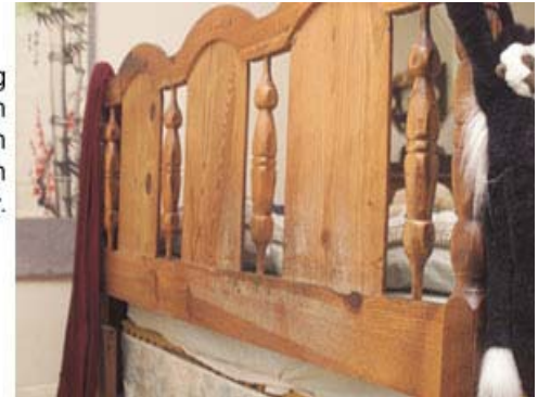
Mold growing on a wooden headboard in a room with high humidity.
